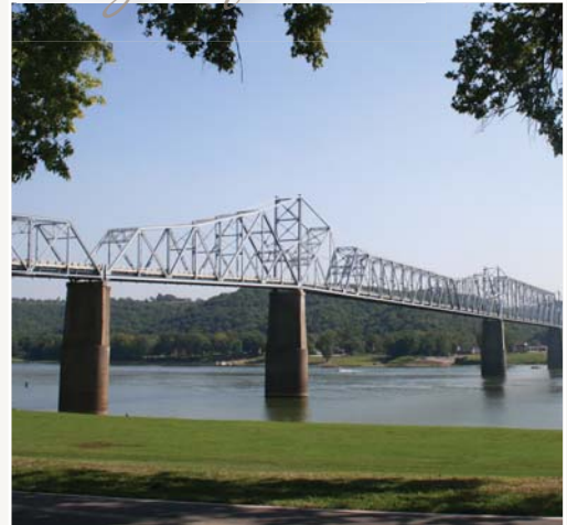
Milton Madison Bridge over the Ohio River between Kentucky and Indiana (photo courtesy Wilbur Smith Associates/Michael Baker Engineers)
